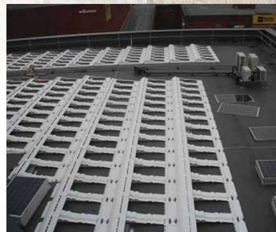
PHOTOVOLTAIC CELLS FOR POWER GENERATION ON SCHOOL ROOF
